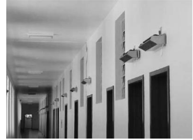
Upper-Air UV-C Devices in TB Facility
