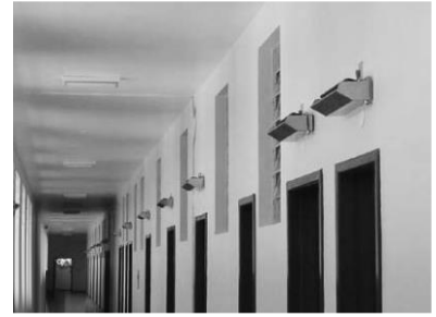
Upper-Air UV-C Devices in TB Facility
