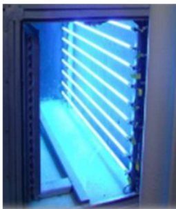
In-duct UV-C system
